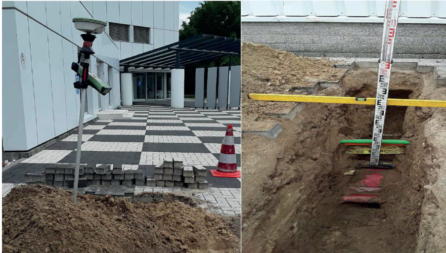
Figure 23. Use of digital GNSS technology (left side) and analog measures (right side) to determine utility locations.
